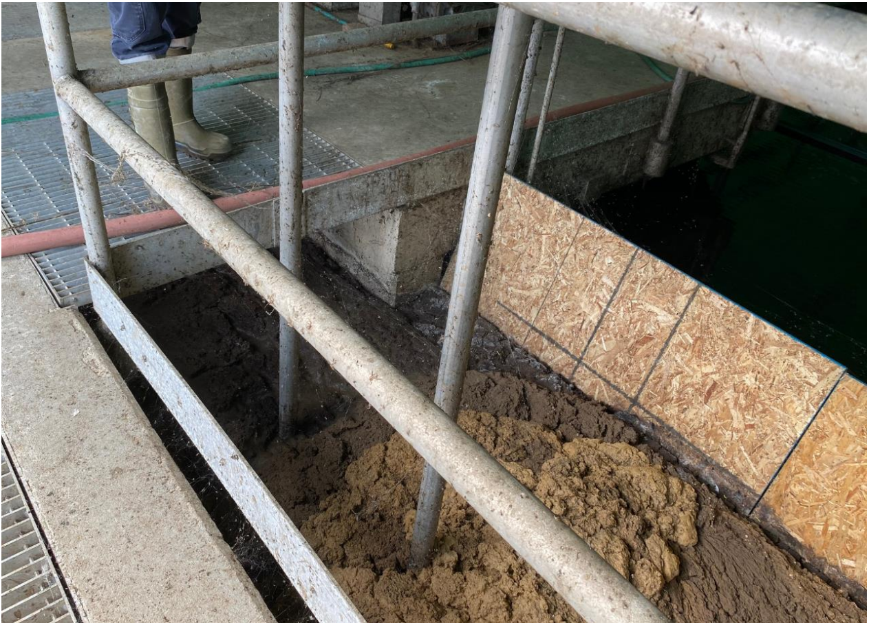
Figure 3 – Temporary Scum / Foam Baffle at Inlet to Secondary Clarifier
