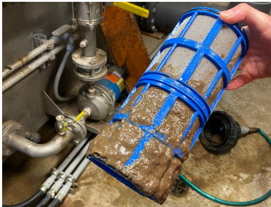
Figure 6 – Canister Filter on Disc Filter Backwash Feed Line
