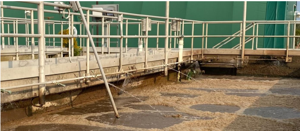
Figure 2 – Effluent Water Spray to for Foam Control
